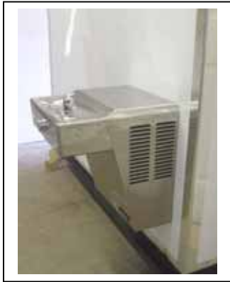
Cold Water Drinking Fountain
